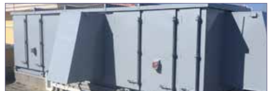
After HVAC New Life
