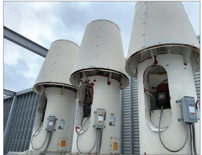
BEFORE HVAC NEW LIFE
