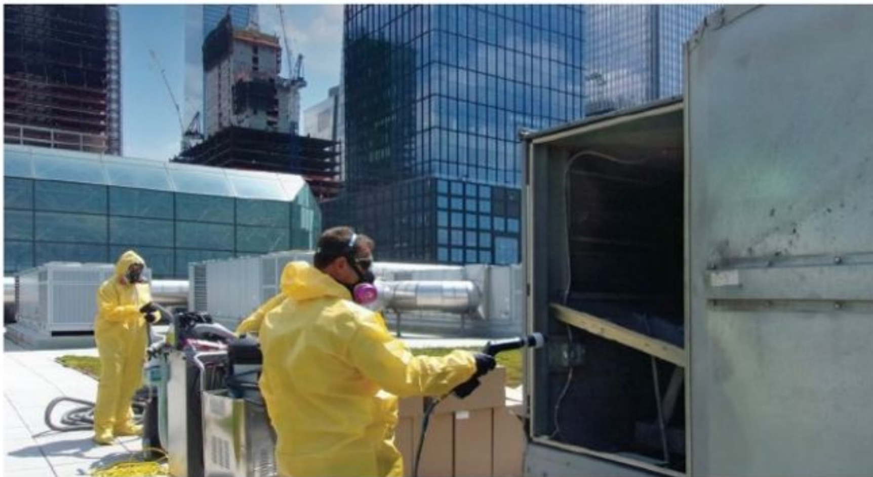
Team working on RTUs at the Javits Center in New York City to restore the over one million square feet of the facility back to civilian use after being used as a COVID-19 field hospital.
