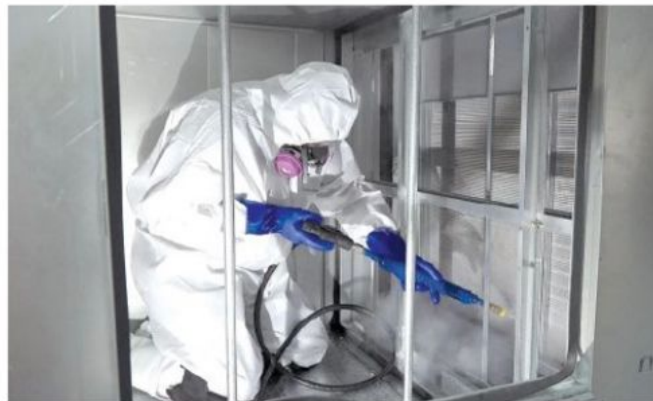
Steam cleaning air handling units in HVAC systems helps to restore performance to near factory specifications, while also helping to lower energy costs.
