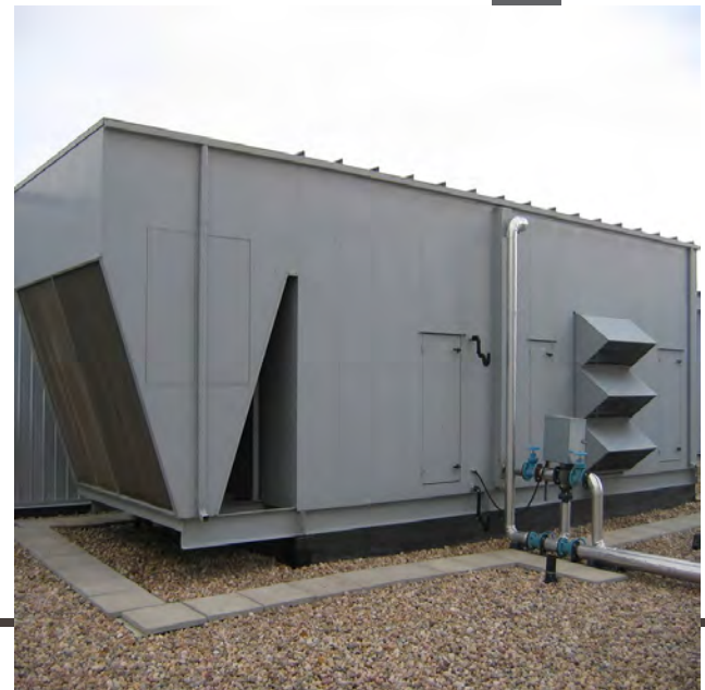
Air Handler Unit
